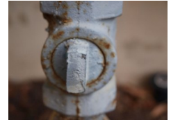
The gas valve is always on the pipe coming up from the ground to the meter on the side of the house. Photo by Emily Peisker
