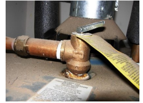
The safety valve can be found at the top or side of the water heater. Photo by Jim Peisker
