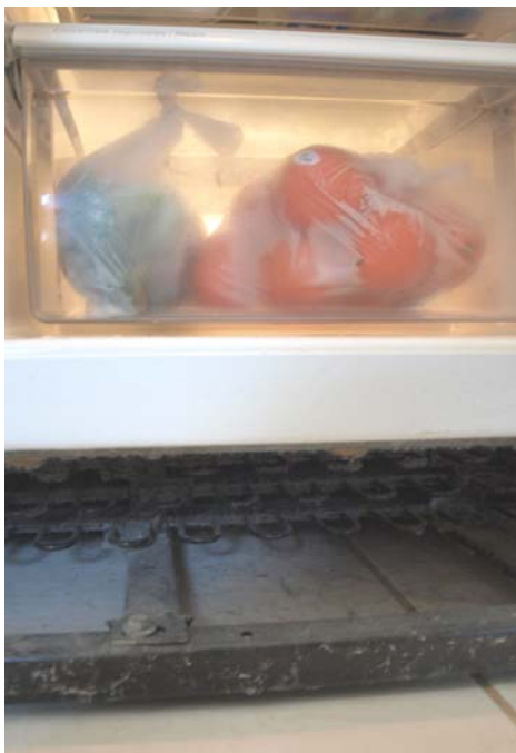
Once you remove the kick plate, you should see one end of several rows of serpentine coils. The basic idea is to get all the dust and dirt out from among the coils without damaging them. Photo by Emily Peisker
